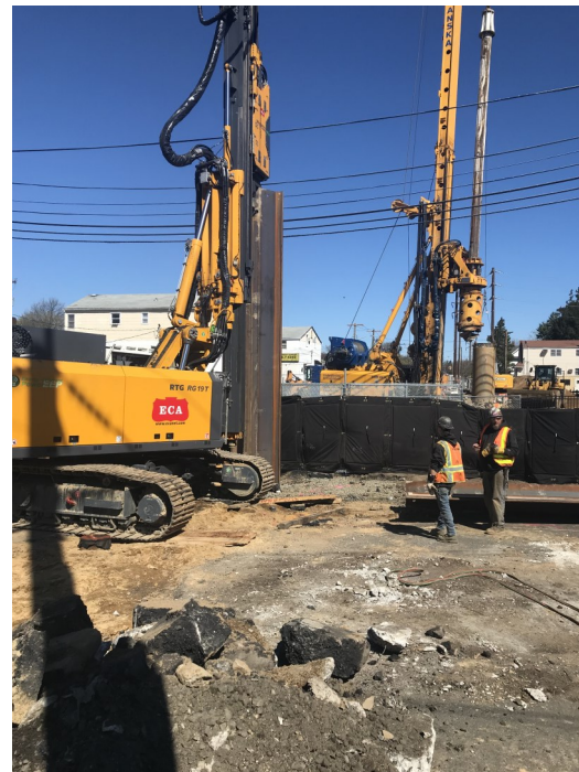
Pile driving is done to support the tracks and keep the earth in place while the construction site is being excavated.
