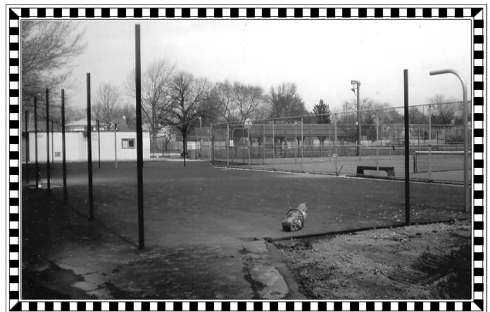
The asphalt paving is completed and next steps include fencing, line striping, and installation of basketball hoops.
