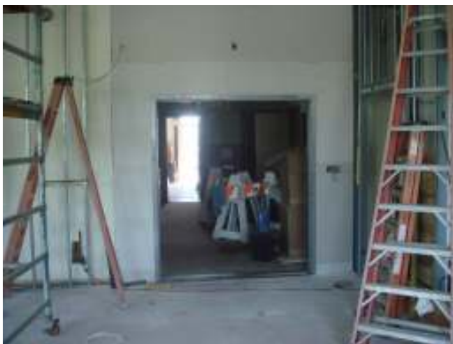
Here's the main entrance to the Theatre. Special fire retardant doors were recently delivered and will be installed soon.
