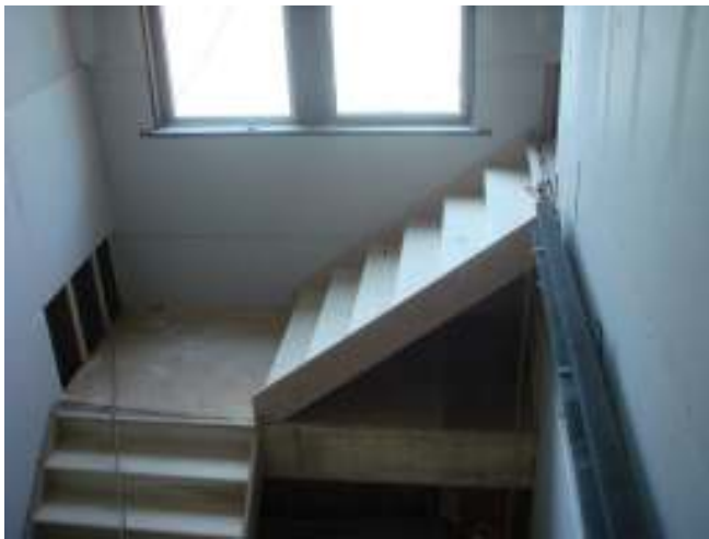
An additional staircase has been installed in the rear of the Theatre.
